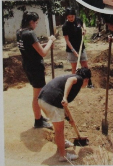
RIGHT: Fintona Girls' School students dig the foundations for a new water system at Akany Avoko, Madagascar.
